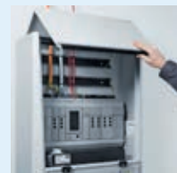
↑ Batterie-/Versorgungssysteme Battery power supply systems
